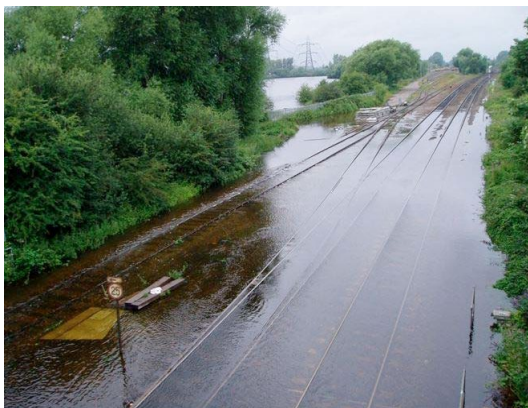
Impact of flooding on transport links – flooding of the railway line north of Old Abingdon Road. July 2013.
